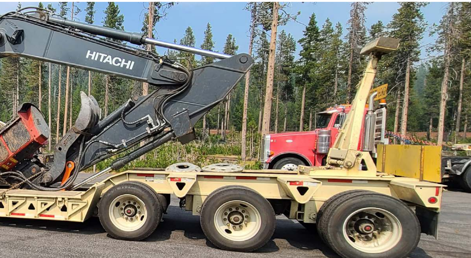
This incident employed large numbers of heavy equipment and had an excellent safety record.
